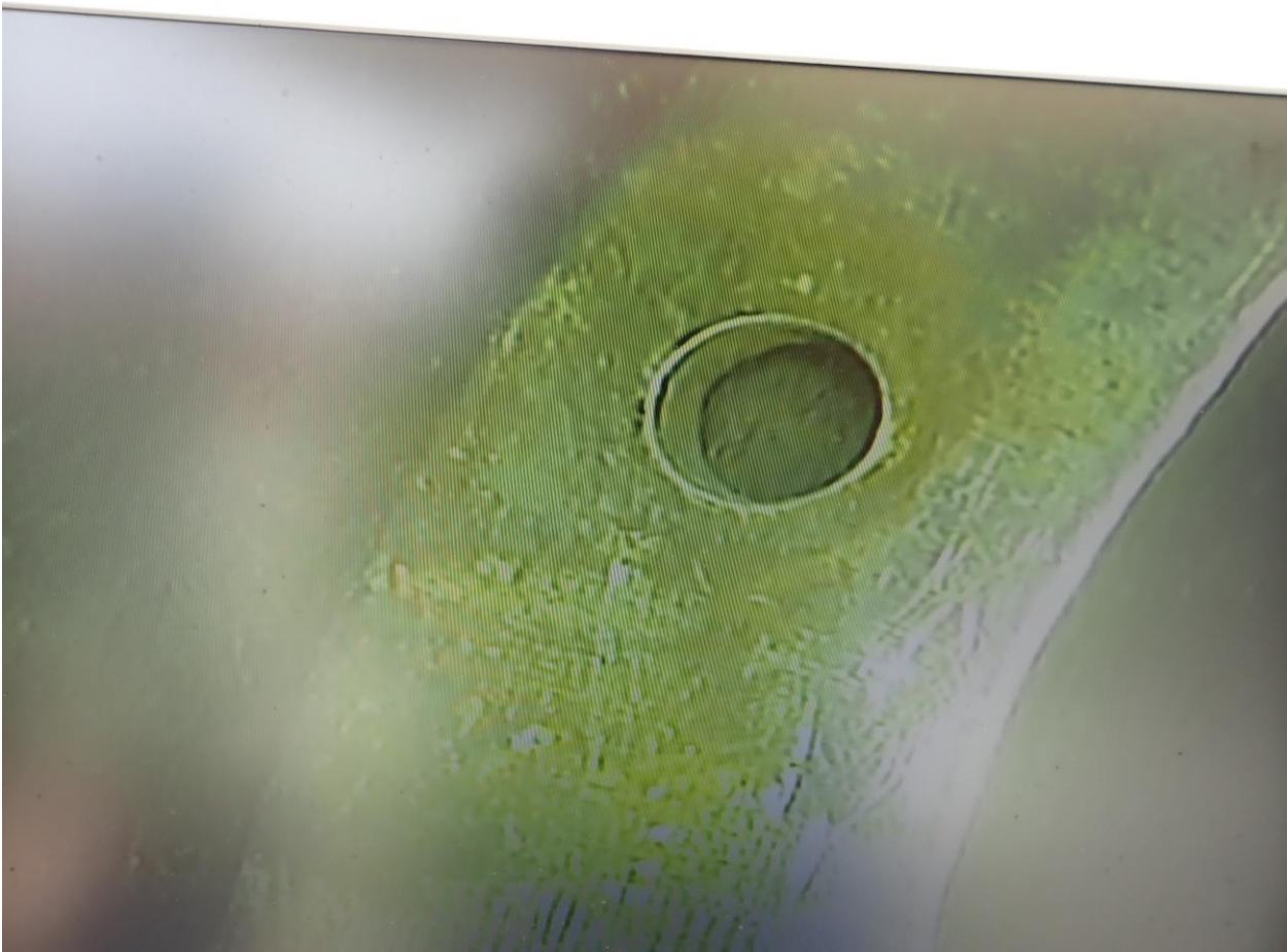
Picture 3: Stainless steel flange with missing bolt found on 6C2, July 9, 2020.
