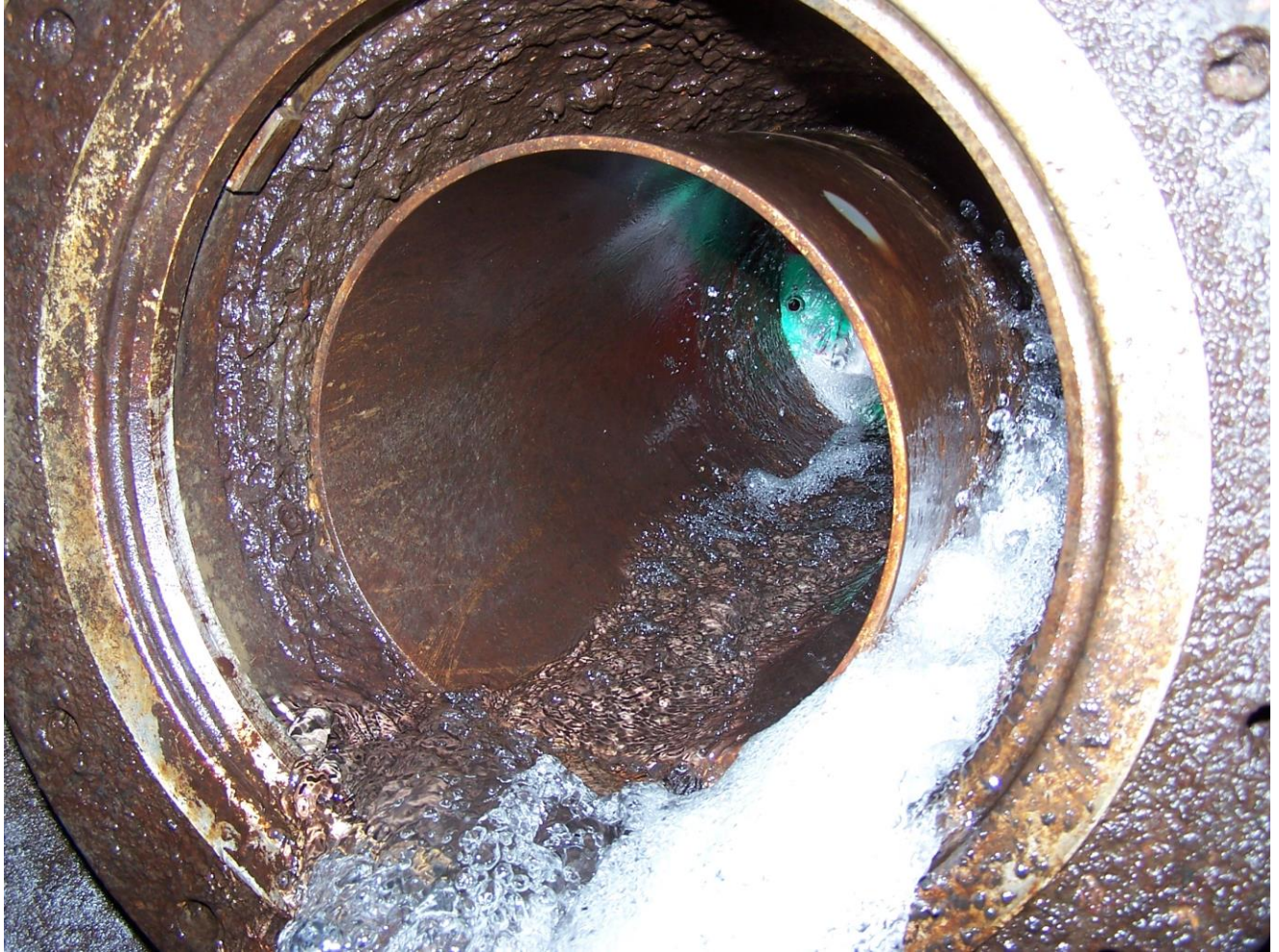
Picture 2: Photo taken looking from the juvenile channel looking toward the gatewell on an unknown orifice from a previous year inspection. You can see the 12" stainless steel liner inside the corroded 16" pipe.
